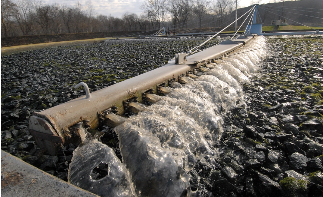
Sewage water runs through a “trickling filter” at Bethlehem’s Wastewater Treatment Plant in this file photo. To discharge its leachate into the Bethlehem Wastewater Treatment Plant, Bethlehem Landfill must receive an “indirect discharge” permit from the city. {Harry Fisher / The Morning Call}
